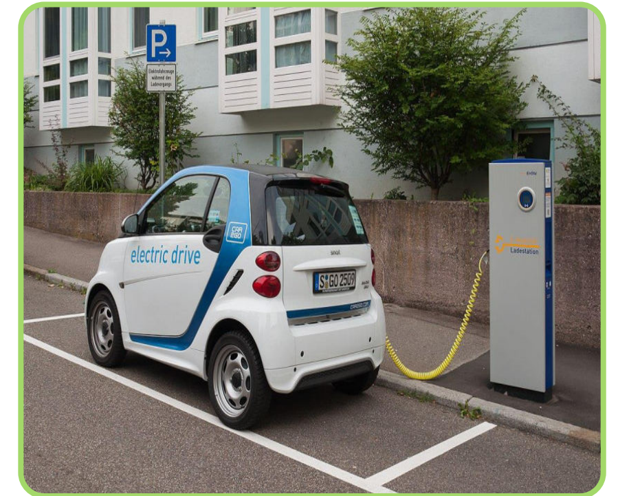
Car2Go Charging Station Stuttgart 2023
